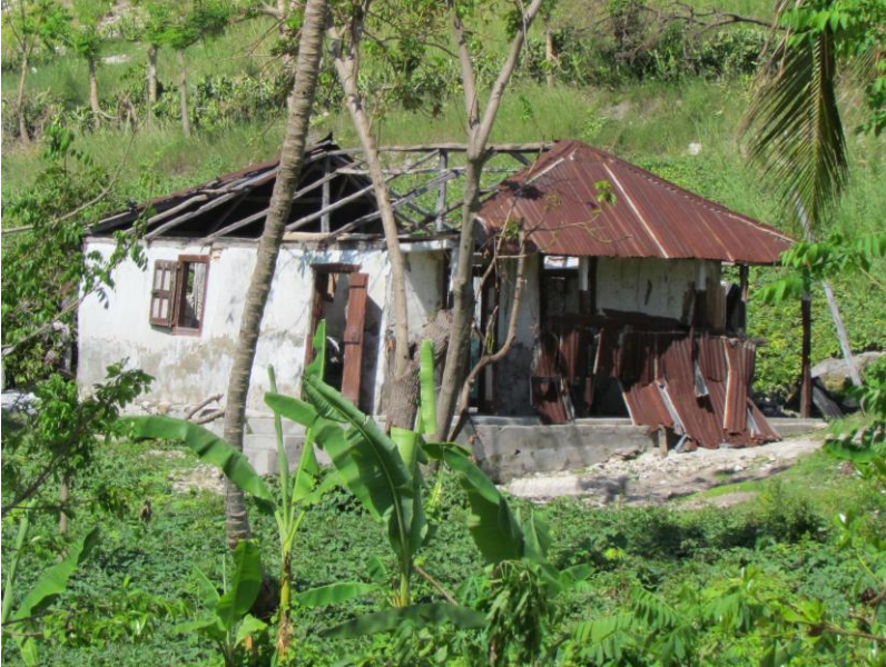
Thousands of homes were damaged or completely destroyed by Hurricane Matthew.
